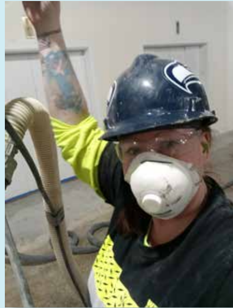
Above: TRAC Graduate and Cement Masons and Plasterers Local 528 member Danyielle Slothaug at work.
